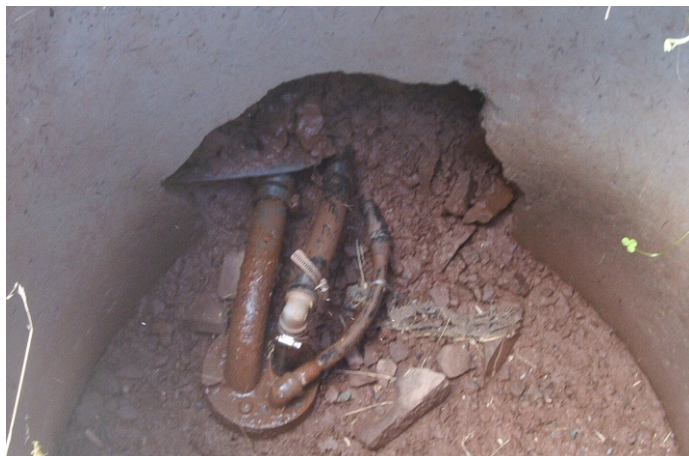
Figure 2: Drilled well cap located in a well pit - to be avoided
